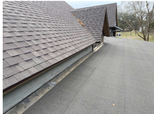
Bannister 7542 Flat Roof 337 SW Koonville Ave • Lake City, FL 32024 Fri, Mar 1 10:03 am by Guillermo Seferino
